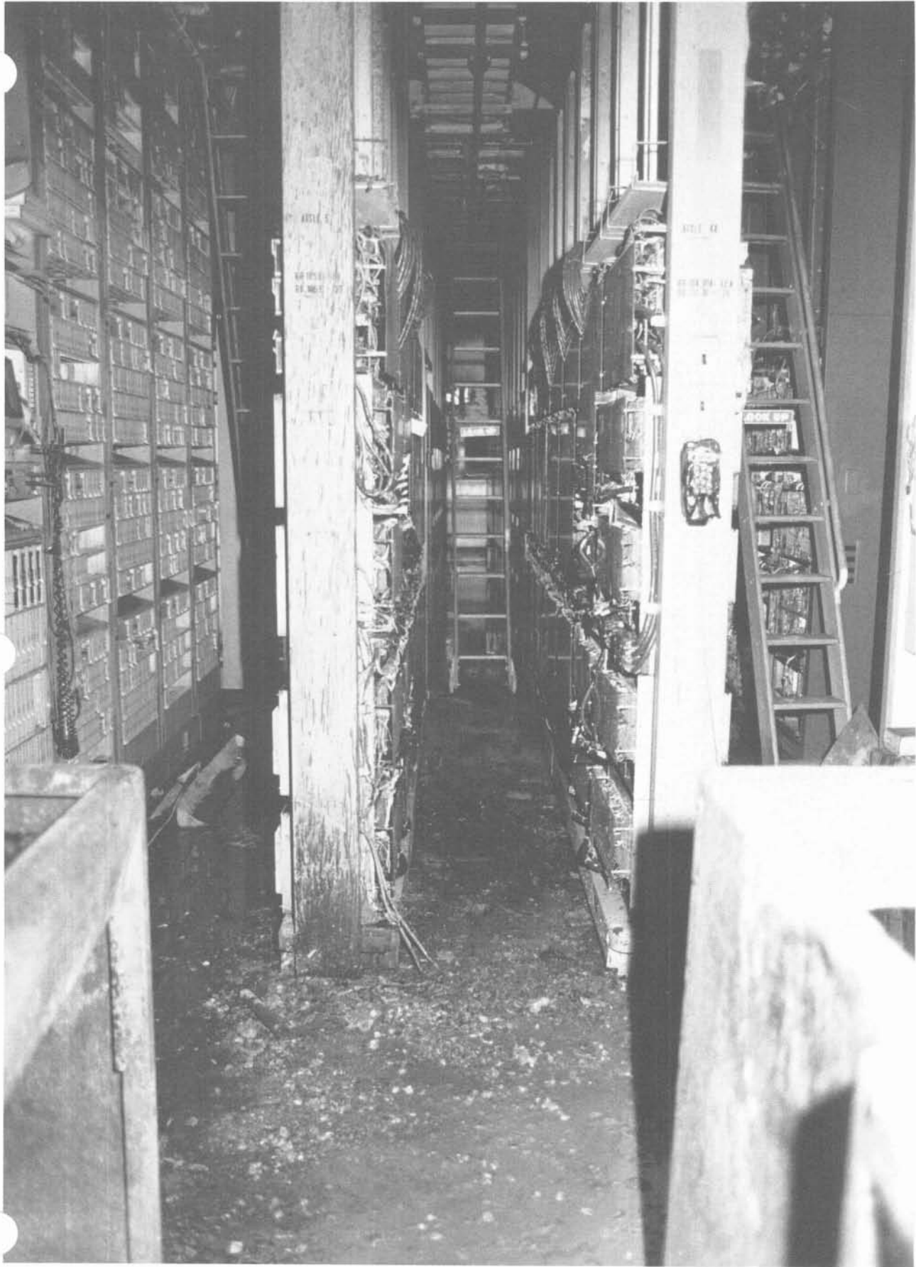
Photograph 3. Fire damage below cable trays shown in Photograph 2.
