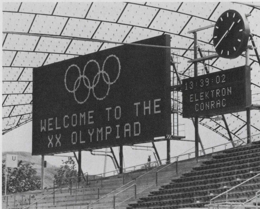
Two giant, computer-controlled displays , designed by Conrac Corp., have been installed in the Olympic Stadium in Munich, the principal site of the Summer Olympic Games. These boards use up to 1.26 MW for operation.
