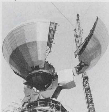
TV signals from the Olympic Games will be beamed around the world from this new earth-station antenna.
