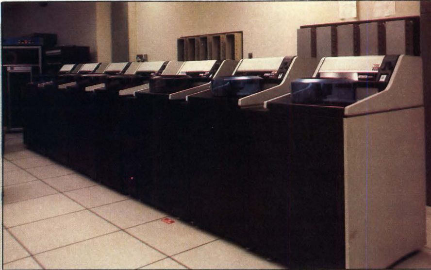
DEC system 10 and VAX 780 computers and DEC rpo6 disk drives are the major equipment in the NNDC main computer room (above). The four magnetic-tape drives are from Storage Technology.
